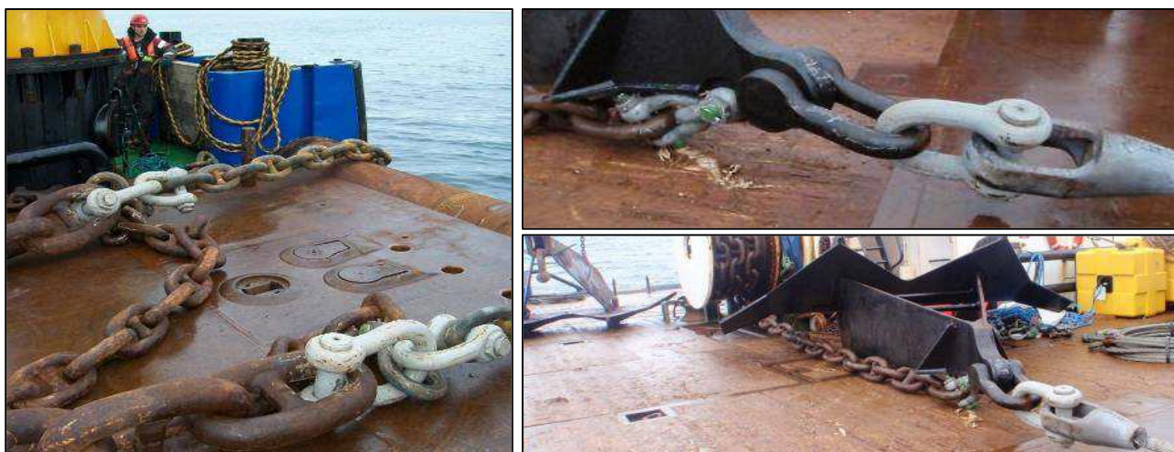
Figure 8: Backup line connection using overrated bow shackle (left) and back to back shackle arrangement used for anchor connection and the majority of chain connection in the mooring system.
