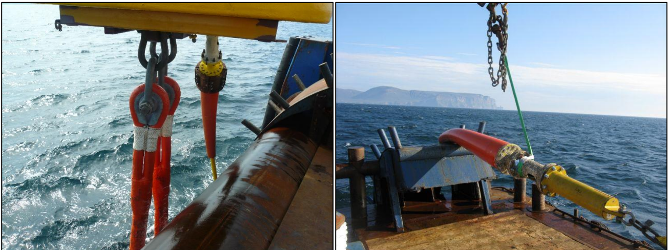
Figure 16: Dynamic bend stiffeners were used at the cable exit point from the TLA (left) and during the cable installation process (right)
